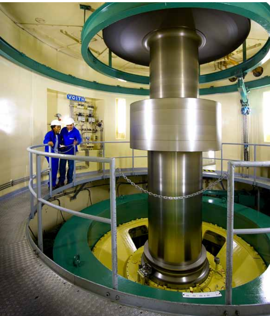
A large motor at the Palmiet pumped storage scheme in the Western Cape
