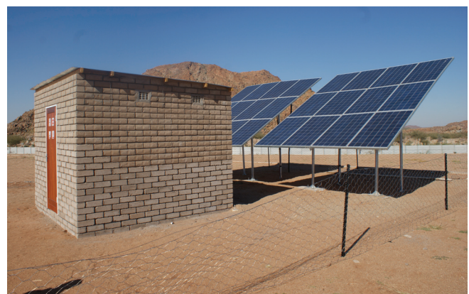
100 solar panels installed in the Riemvasmaak pilot project
