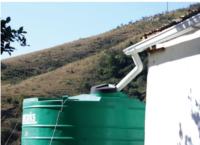
Rain water harvesting in Msinga
