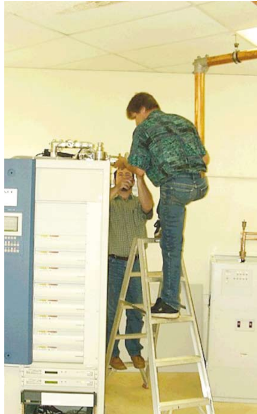
Sentech technicians working on a digital transmitter
