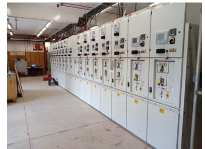
Tygerberg Hospital – 11kV Generator Panel Upgrade
