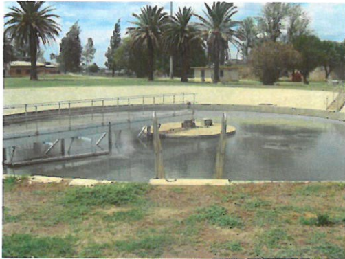
Figure 3 – Primary settling tank
