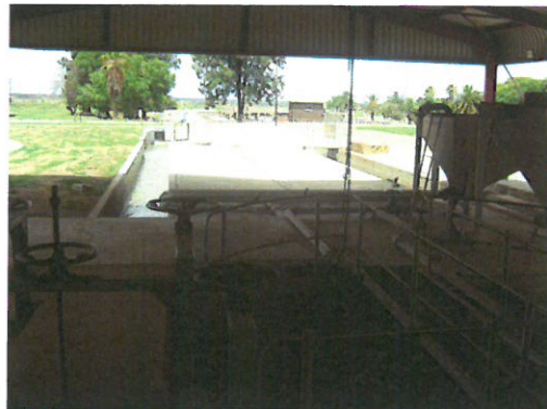
Figure 4 – Grit removal not taking place
