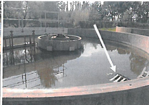
Fig10: Settling tank (material floating)
