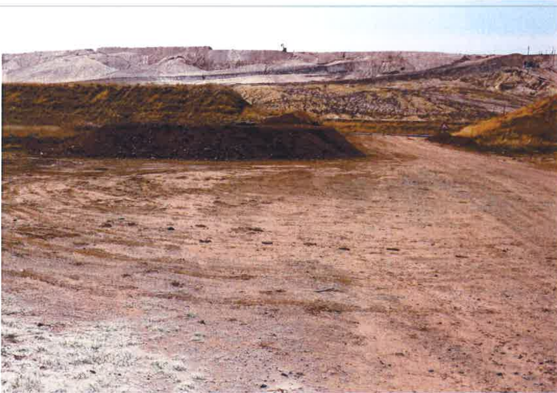
Figure 15: Clean storm water diversion culvert at entrance to Kareerand TSF
