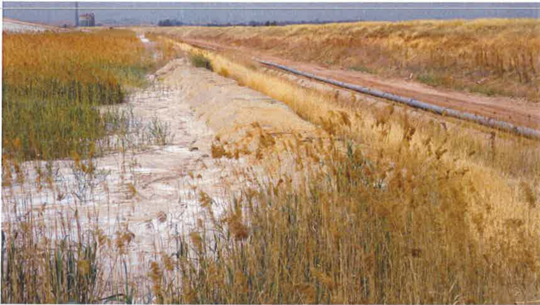
Figure 13: Toewall at bottom TSF sideslopes
