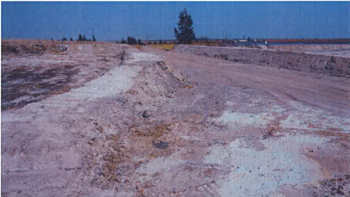
Figure 18: Temporary storm water containment next to return water dams (till East Storm Water Dam constructed)
