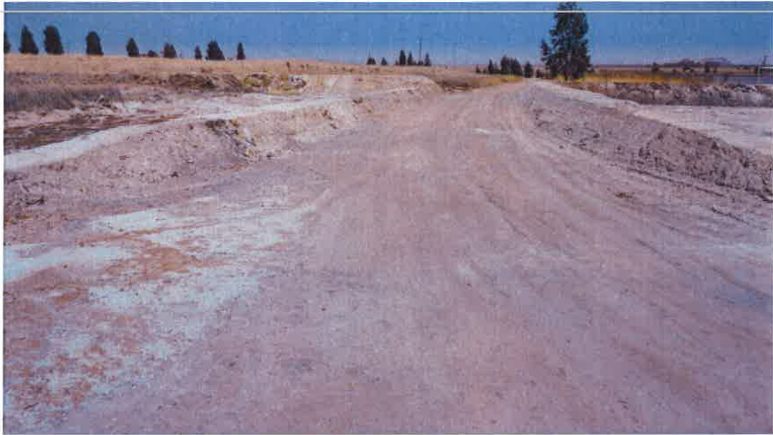
Figure 17: Temporary storm water containment next to return water dams (till East Storm Water Dam constructed)
