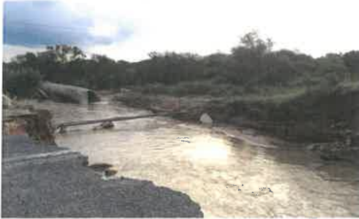
Figure 4: Road washed by 2014 floods in Vaalwater
