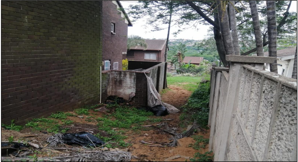
Figure 4-8: Signs of downhill erosion at 2 Periwinkle Garden along 49 Etterick Road's Boundary fence
