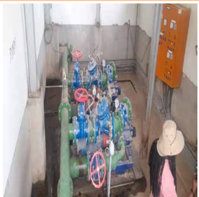
Figure 45: Damaged pumps and electrical at Mangxamfu water
