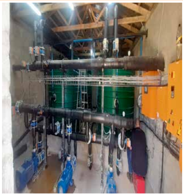
Figure 47: Water purification plant at Humansdorp
