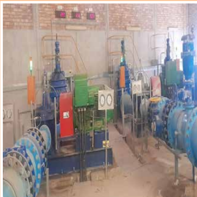
Figure 44: Water pumps inside the Motherwell pump supply
