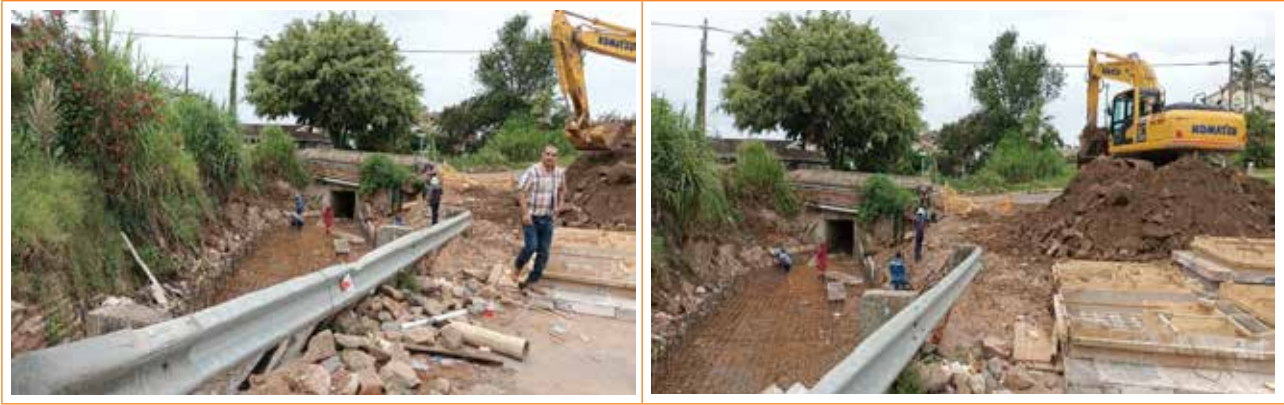
Figure 41: Syringa drive Chatsworth Construction of a concrete canal and laying of a stormwater pipe as well as construction of stormwater manholes (eThekwni, KZN)
