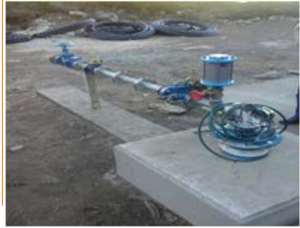
Equipped borehole ready for production
