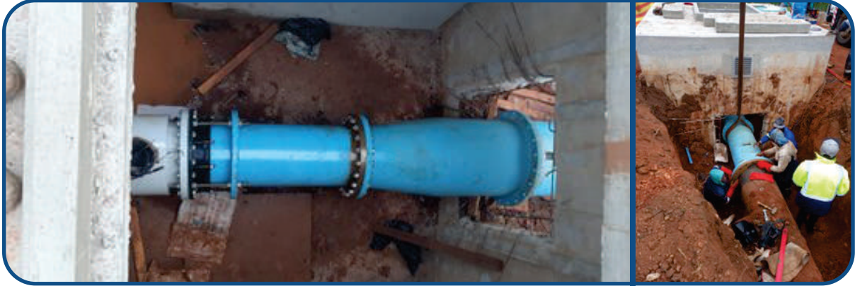
Ebenezer installation of a new balancing flow meter and manhole within the Ebenezer Water Scheme
