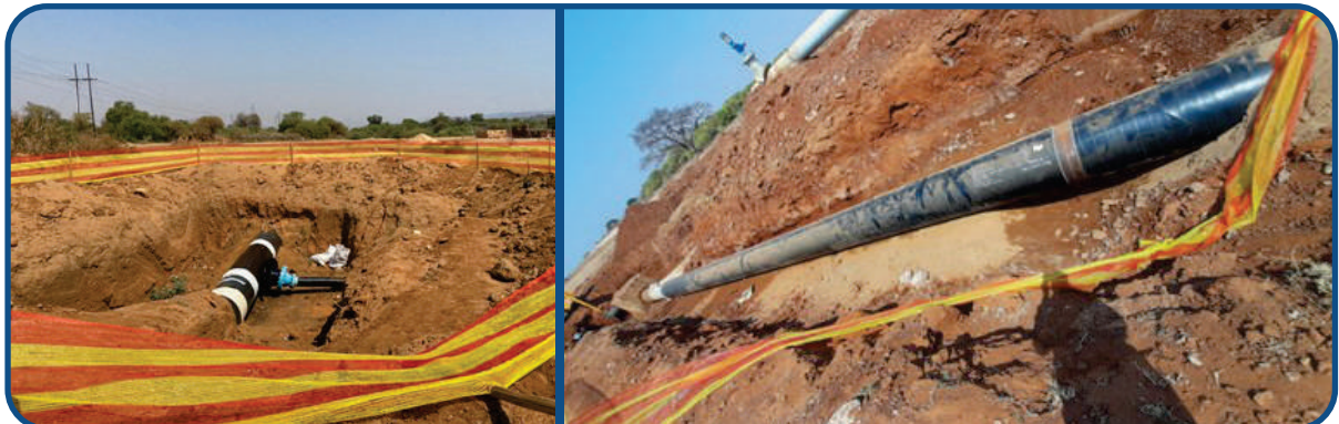
Replacement of the Specon Phase 2 – 2,4 km bulk pipeline within the Olifantspoort Scheme
