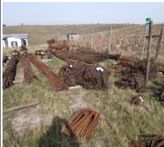
Material on Site: Steel reinforcement for 1ML Reservoir roof and 500 kl Reservoir. G5 layer works
