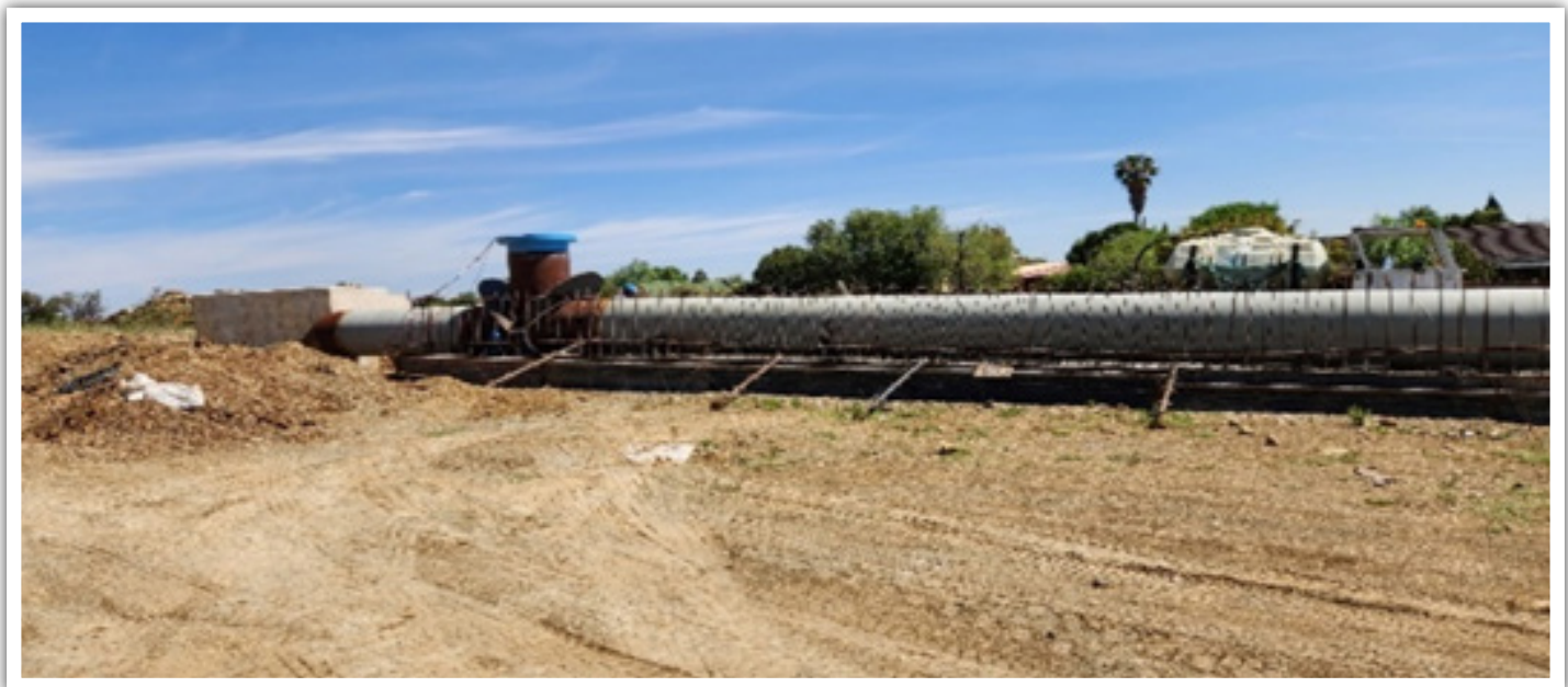
Construction of the steel pipeline and related infrastructure from the Welbedacht Dam to Bloemfontein
