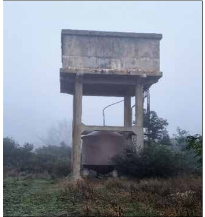
Cement holding tank which is the main holding tank for water from the Wemmershoek scheme. Water from the borehole can be pumped from the tank.
