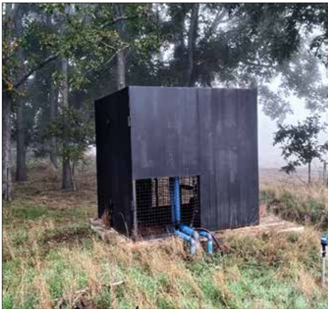
One borehole enclosed in the metal cage. This is also the combined pumping facility where the two boreholes' electrical controls are and where their delivery is combined. Each borehole can be operated separately.
