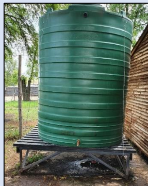
Steel stand for water tank at Jabula Combined School not level
