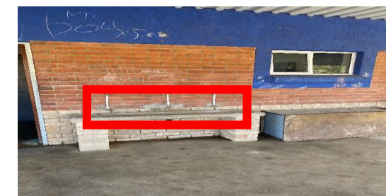
Figure 7: Eyabantu SSS Missing taps due to vandalism
