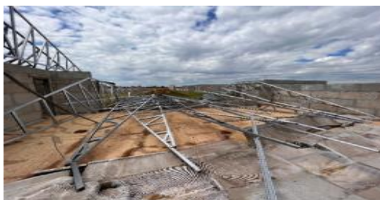
Figure 3: Loretlweng PS Collapsed roof trusses and walls
