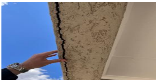
Figure 2: Tlotlang Thuto Cracks on the edges of the structure.
