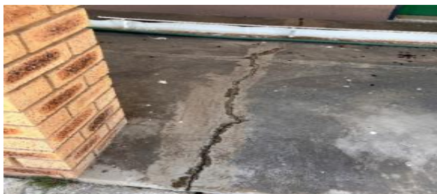
Figure 1: Tlotlang Thuto - Cracks in the walkway
