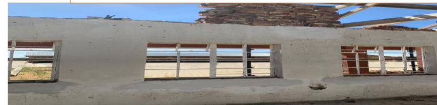
Figure 5: FS Tshehetso Primary Poor workmanship on brickwork and plastering.
