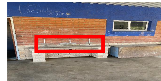
Figure 7: Eyabantu SSS Missing taps due to vandalism
