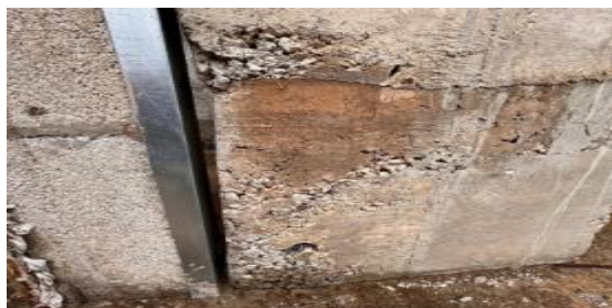
Figure 4: Loretlweng PS Gap between Green Crete wall and the concrete wall
