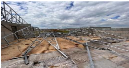
Figure 3: Loretlweng PS Collapsed roof trusses and walls
