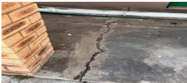
Figure 1: Tlotlang Thuto - Cracks in the walkway
