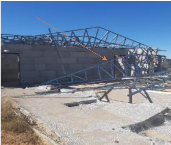
Figure 7: Collapsed roof trusses
