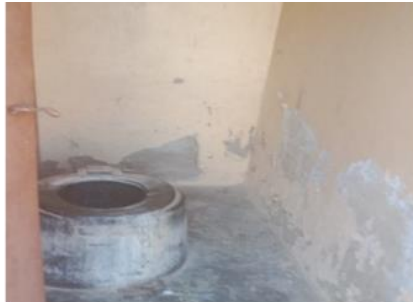
The nature of abluion facility at the Siligane School in MP
