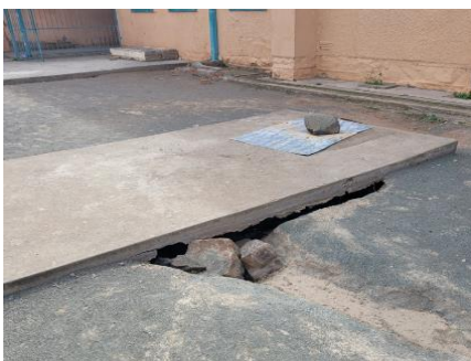
Unattended manhole at the Phakamisani School in NC
