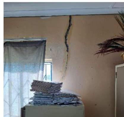
Structural cracks at Banzana High School in KZN
