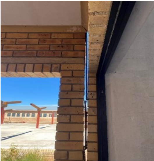
Figure 15: Visible gaps & openings in brickwork
