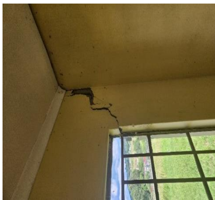
Structural cracks at Maqhingendoda Secondary School in KZN
