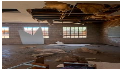
Damaged ceiling at the Sebalamakgolo School in LP
