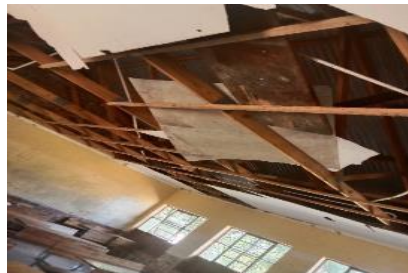
Damaged ceiling at the Siligane School in MP
