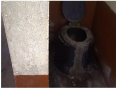
Filthy toilets with no doors at the AV Plaatjie SSS in EC
