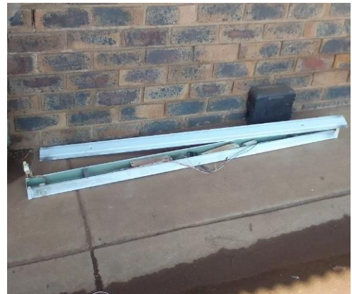
A broken lamp with exposed electrical wires at Tlhoafalo primary school NW
