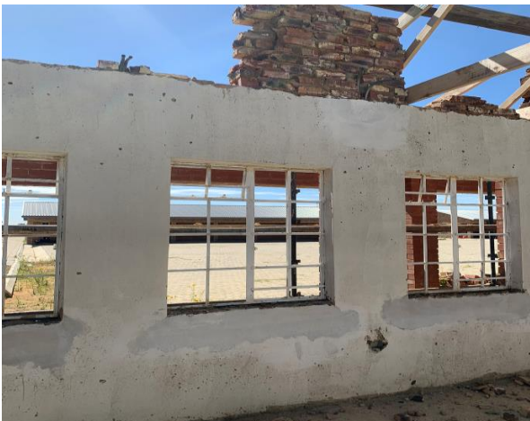
Figure 13: Poor workmanship on brickwork and plastering removed
