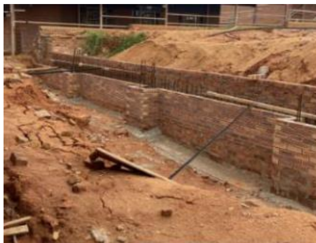
Figure 6: Retaining wall collapsed and not rebuilt or properly barricaded off
