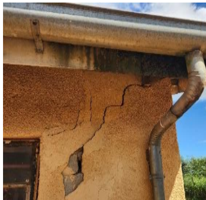
Structural cracks at Langeni Combined school in KZN
