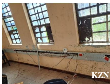
Exposed electrical wires inside classrooms captured at Banzana High School in KZN
