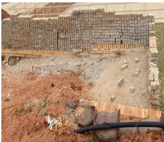
Figure 5: Paving stacked on walls – dangerous
