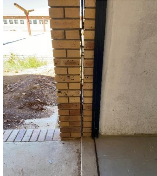
Figure 16: Visible gaps & openings in brickwork
