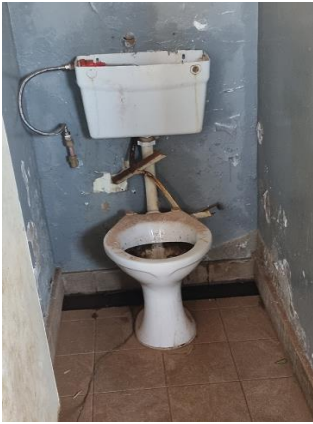
Figure 3: ablution facility not age-appropriate at Bakang Primary
