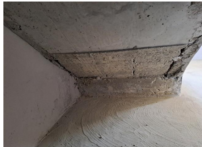
Figure 1 & 2 : Cracks on honeycombing underneath the staircase
