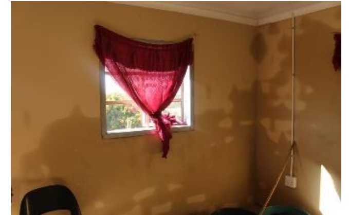
Figure 3: Water penetration on internal walls
