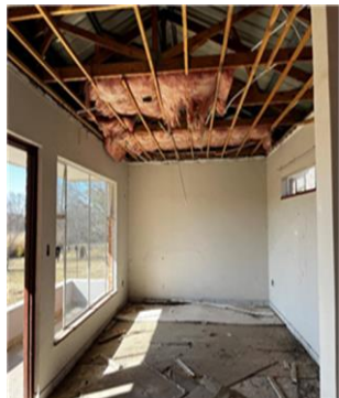
Peeling due to high moisture
