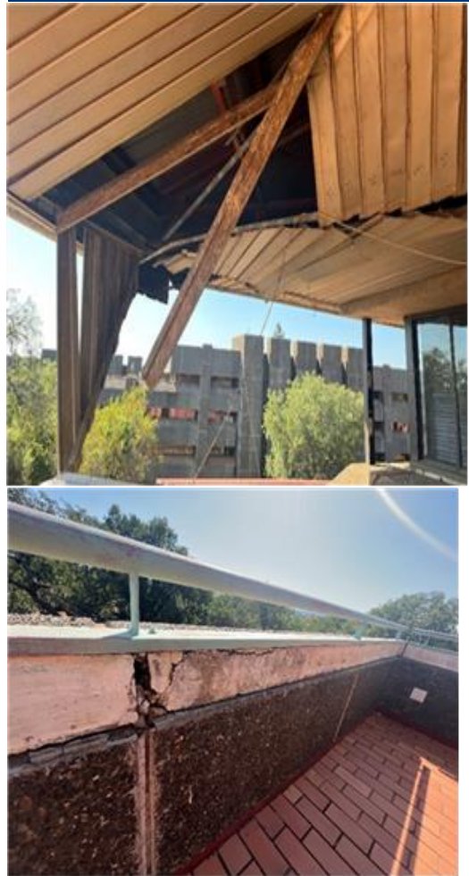
Example of building visited by the AG team at Old Parliamentary Village
