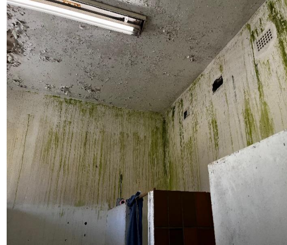
Mould and moisture forming on the kitchen cell wall and paint peeling from the slab
