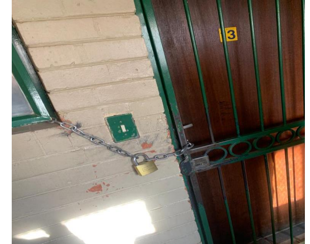
This is the door to the firearms room (storage) and the handles are not working hence this method of chain and lock is used .
