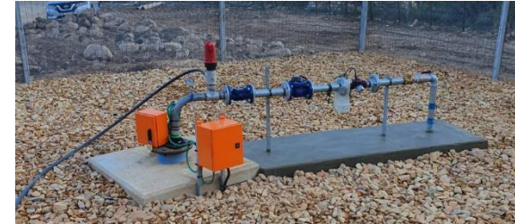
Telemetry System Upgrade (Beaufort West)
