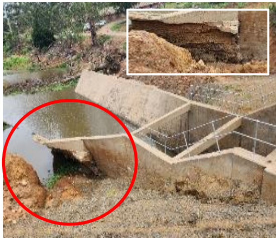
Wall used to channel water downstream had no fill material and appeared to be collapsing (inset)
