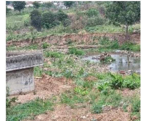
Close proximity of treatment works to river, with no risk reduction measures instituted to prevent ingress of water if river level rises
