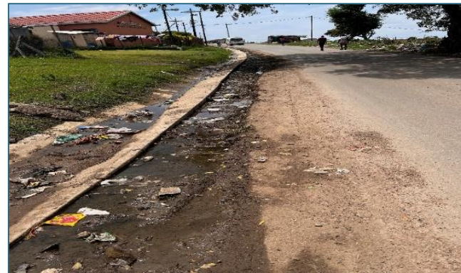
Nkobongo road – Recently repaired road with incomplete area between V-drain and road
