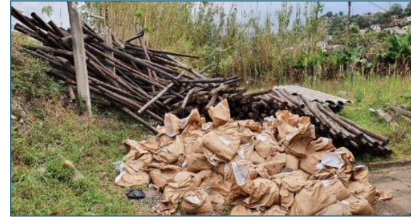
Building material purchased left exposed to weather elements at Umlazi mass care centre
