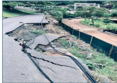
Road damaged by floods without warning signage or markings to inform public (Wood Road)
