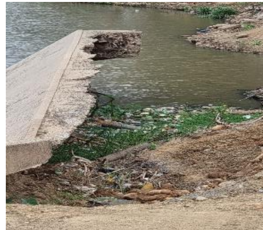
No fill material to support concrete channel
