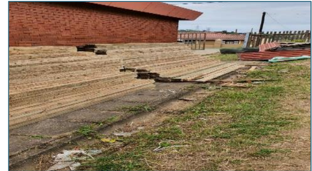
Building material purchased left exposed to weather elements at Umlazi mass care centre
