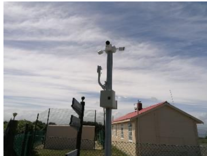
Fig 2: CCTV at village precinct
