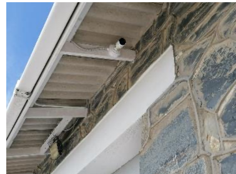
Fig 3: CCTV at MSP and Harbour precinct
