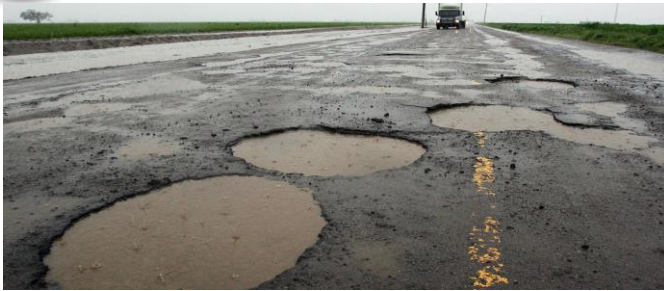
Free State Agriculture (FSA) has warned that the Free State province's road infrastructure is in a dire state.
