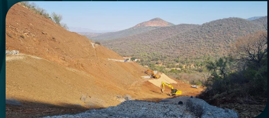
Top: Construction of storm-water control channels and blankets at Uitval Asbestos Mine in Limpopo Province.
