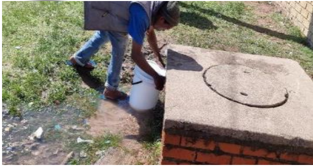
Overflowing manhole used as source of water in KwaDabeka
