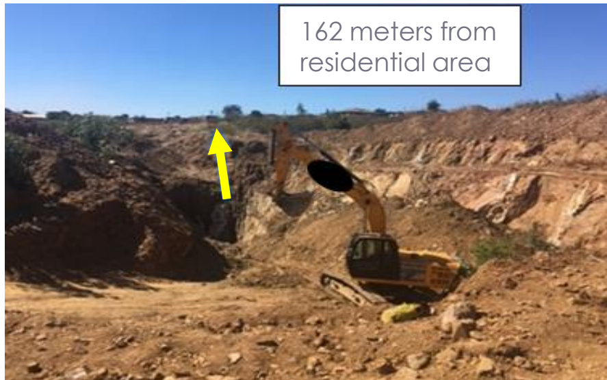
Active mining on previously closed holing site close to residential area in Limpopo
