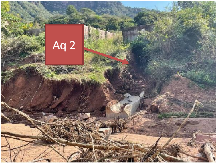
Site Location 3A- wash-away of Aq 2
