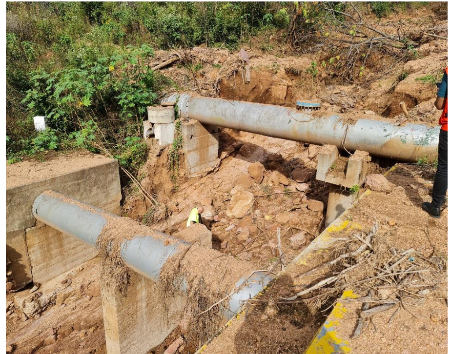
Site Location 2- damage to the foundation of the supports
