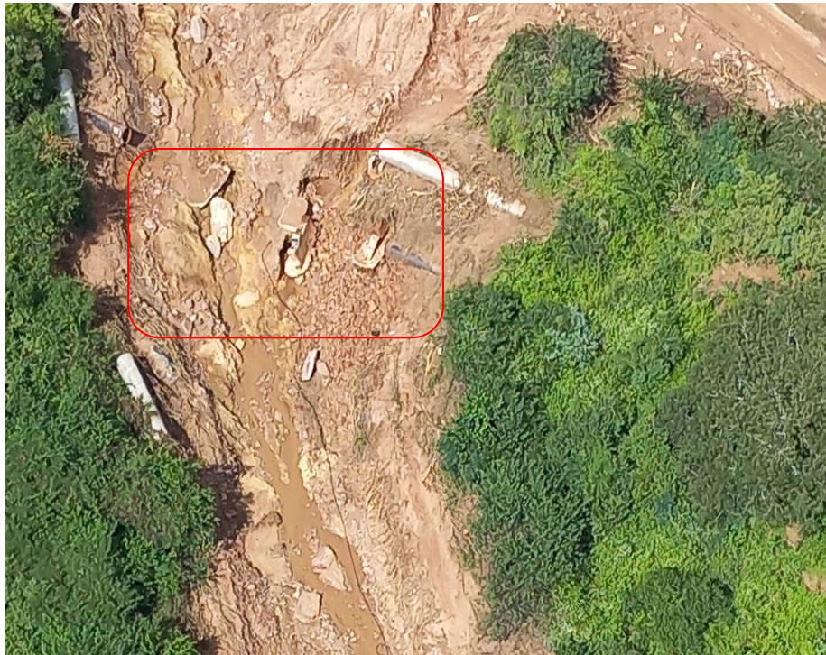
Site Location 1- Complete wash-away of aqueducts 1 & 2
