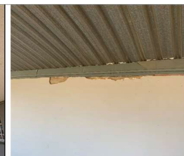
Picture 2: Damaged upper wall Eastern Cape)
