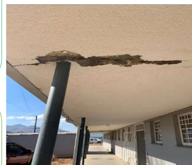
Picture 1: Concrete slab joint damaged (Eastern Cape)
