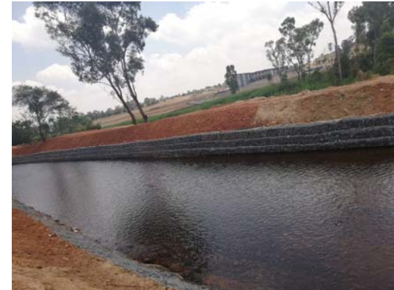
Completed Van Ryn Canal in East Rand (Gauteng Province) for ingress control
