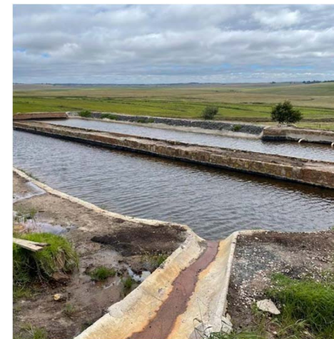
Passive treatment pilot plant in Carolina (Mpumalanga Province) for acid mine drainage remediation
