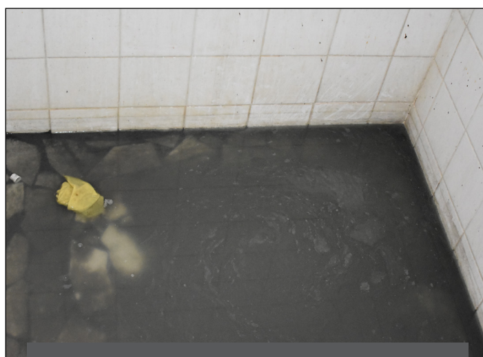
Stagnant water in one of the dormitories in Molehe Mampe
