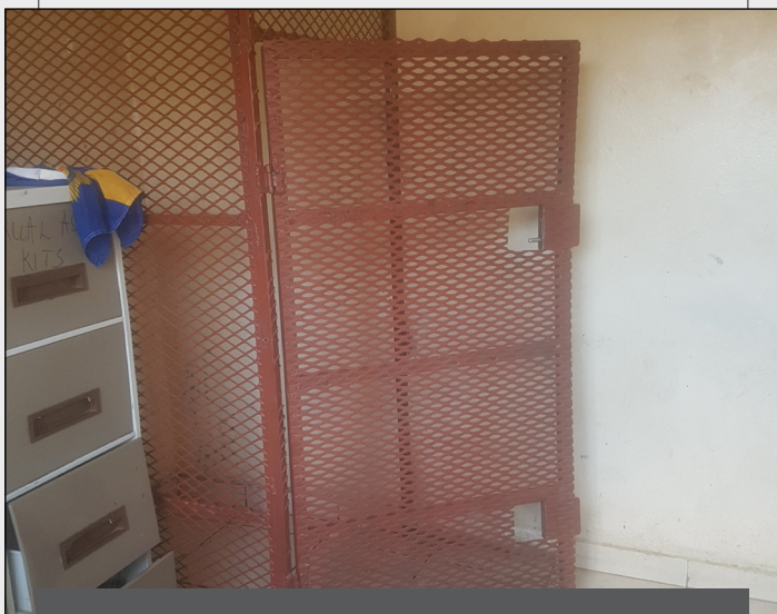
Sebayeng police station was found to be of poor quality
