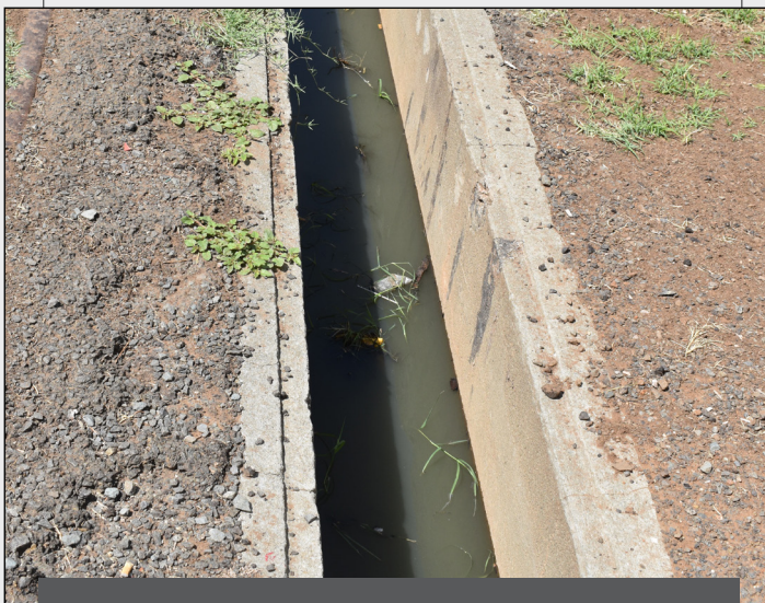
Sewage running through a police facility in the Northern Cape
