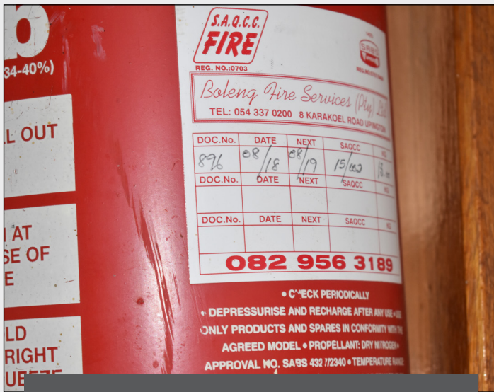
Expired fire extinguisher
