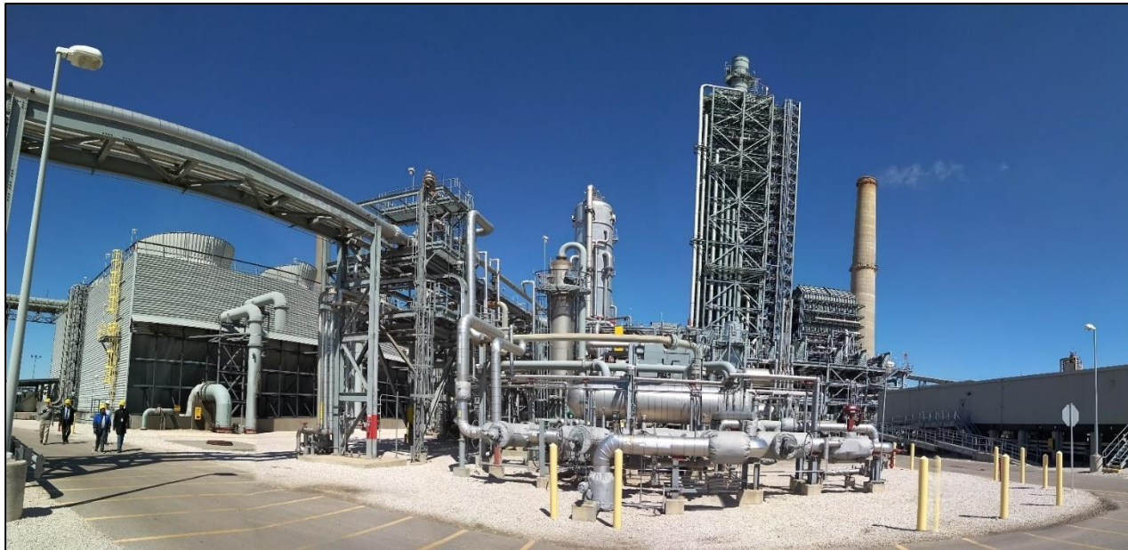
Petra Nova CCUS plant, USA. Captured CO 2 is extracted during the generation of 4,600 MA of energy and the captured CO 2 is utilised toward enhanced oil recovery.
