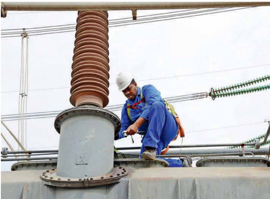
Maintenance at the Apollo substation, the only high-voltage, direct current substation in South Africa
