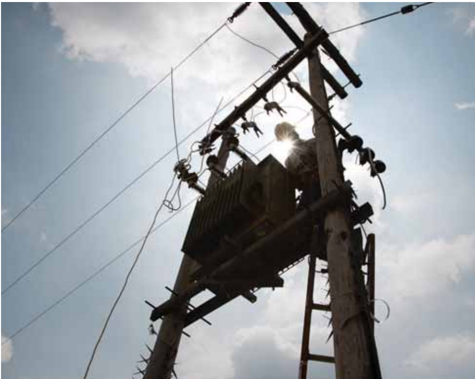
A typical distribution line in the Cullinan area
