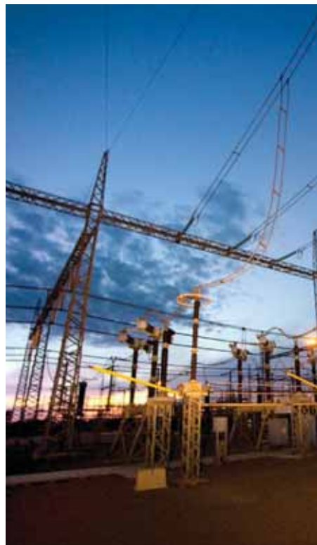
Apollo substation in Johannesburg is the main interconnector to Cahora Bassa in Mozambique
