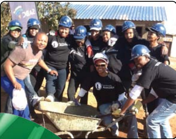
SABC partnered with Habitat for Humanity where SABC staff members built three houses for the families of Orange farm.
