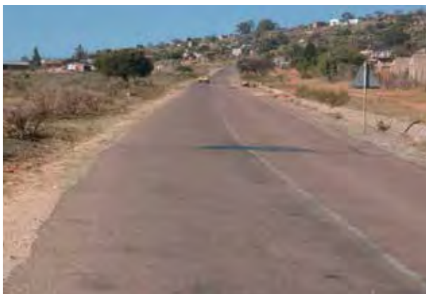
A rural access road in Limpopo, where CSIR recommendations on rural roads have been implemented.
