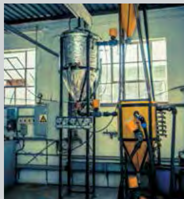
A biogas digester which breaks down biological waste.
