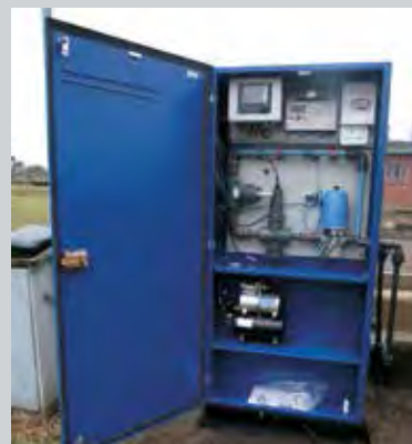
A real-time monitoring system for wastewater.
