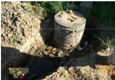
Typical Blocked Soak-away
