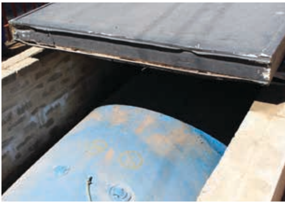
Figure 18: Operational Biogas Digester at Tygerkloof Combined School.
