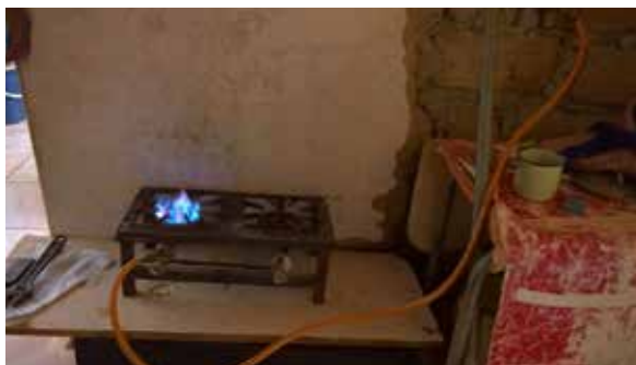
Figure 16: One of completed and operational biogas digester systems operational in Mpfuneko Village.
